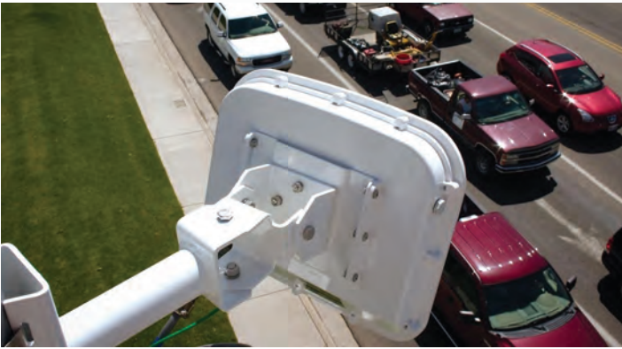
Figure 4-6: Example of a Vehicle Detection System
