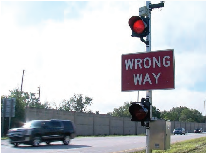
Figure 7-8: Interstate Field Devices and Systems
