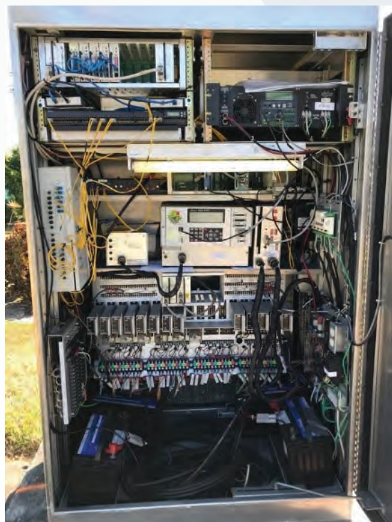
Figure 7-7: ATMS Field Devices and Systems
