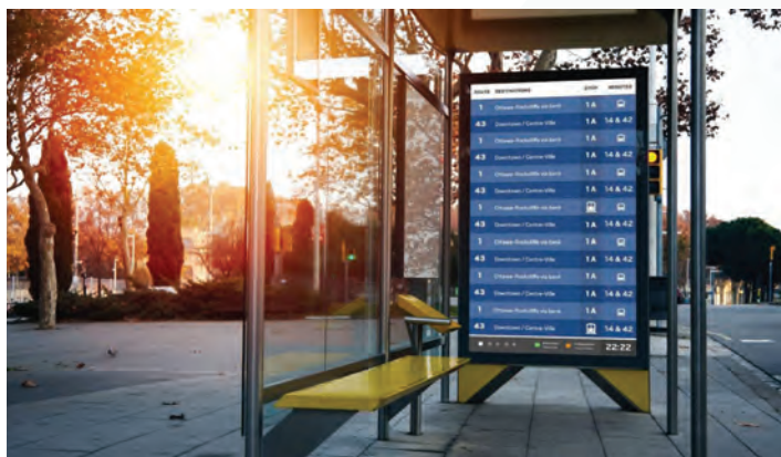
Figure 7-11: Transit Field Devices and Systems
